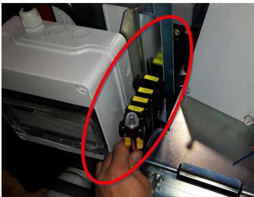
12V system fuse
