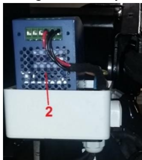
2 = Converter 230V AC/ 12V DC
