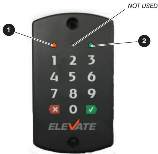
Figure 05 Keypad of the access control unit
